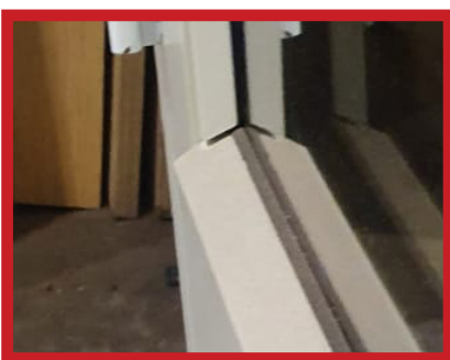
Jamb bead cut short, with bottom bead and seals connecting with glazing to ensure water cannot run in through bead joints
